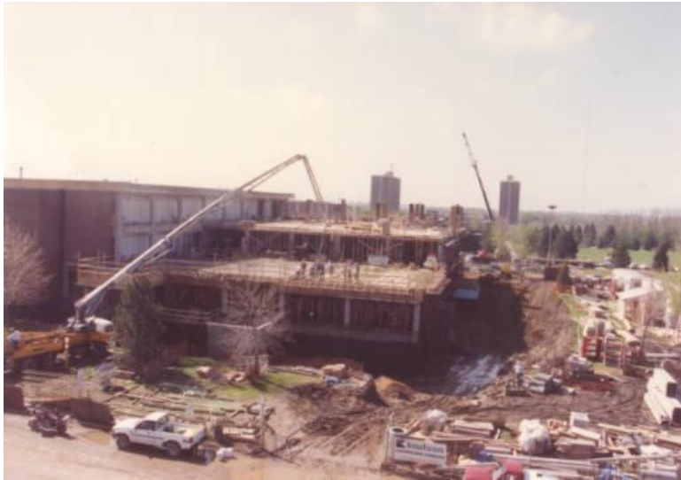
A photograph of the construction on Memorial Library addition; Unidentified workers on building; Mankato State University, 1991.
